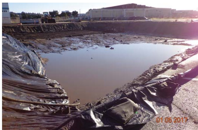
Stormwater in the chlorinated solvent area soil excavation at IR17 and Building 503 Area SWMU 78 and Building 505 Site
